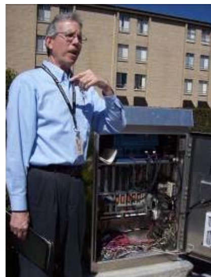
Richard Nassi shows the inside of the traffic signal controller at the Fellowship Square/ 8200 East Broadway Boulevard signalized HAWK pedestrian crossing to the audit participants.
